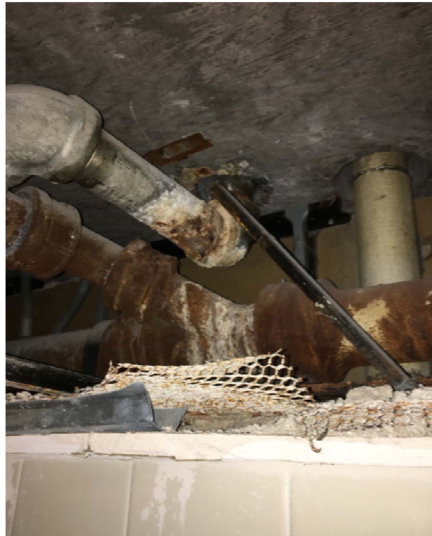
Deteriorating shower vent
