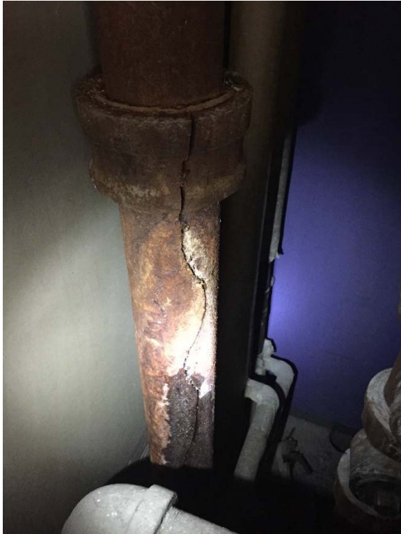
Cracked sanitary drain riser in the wall
