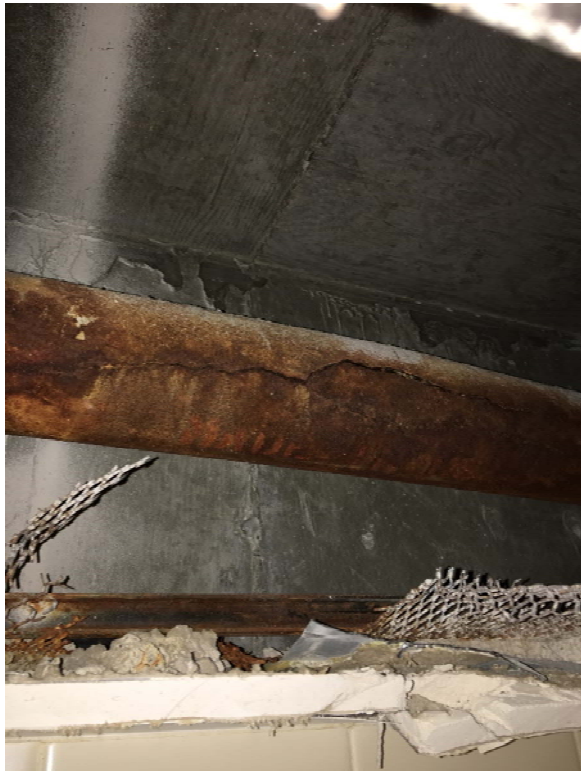
Cracked horizontal drain line above the ceiling
