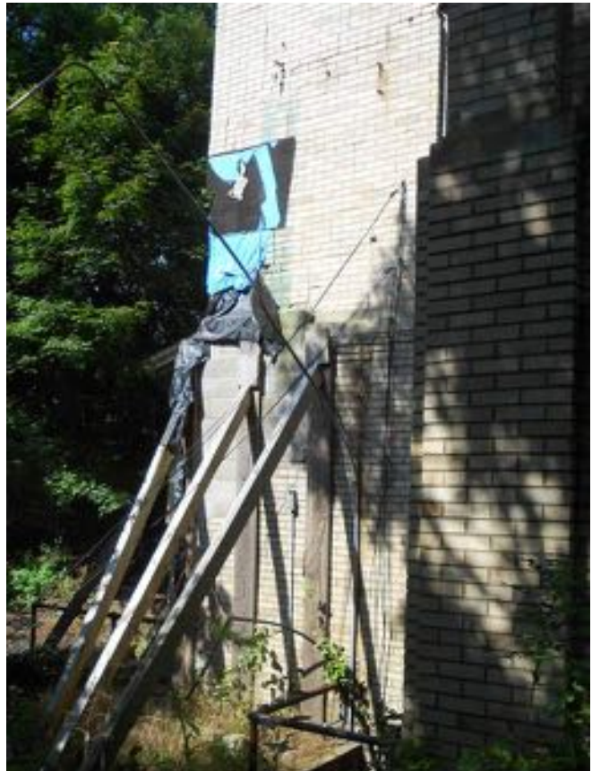
POOR BUILDING CONDITION ON UPPER SOUTH CAMPUS
