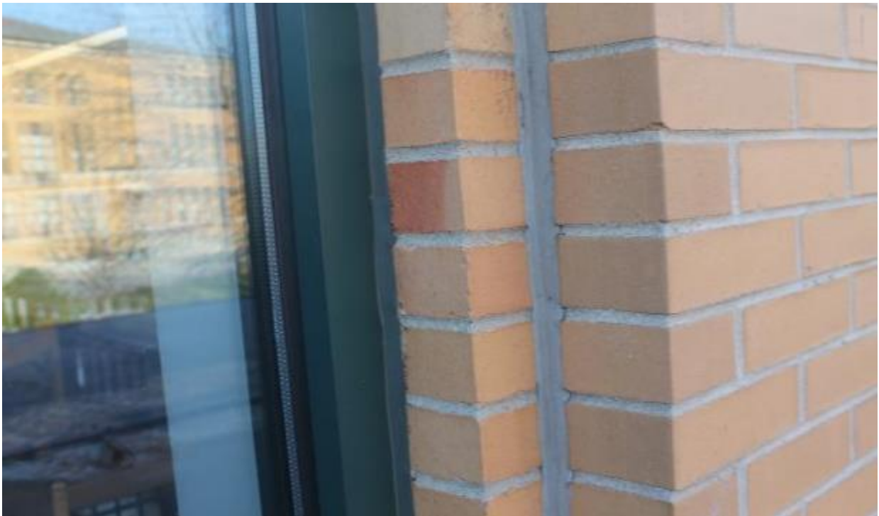
Photo 6: Black window caulk and grey seam caulk on connector roof
