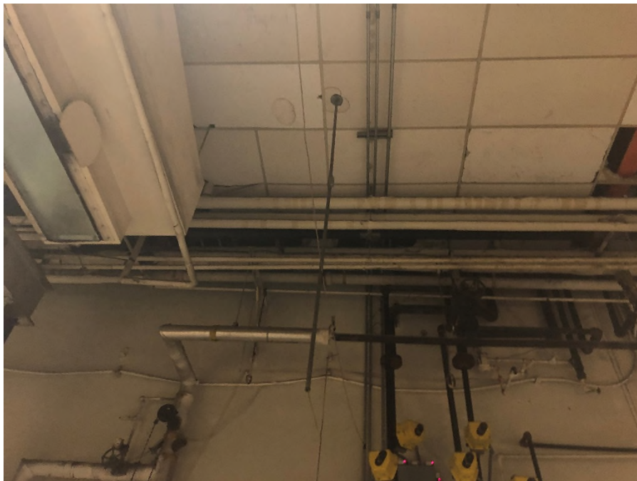
Boiler Room. Note 2'x4' crow feet ceiling tile and ACM pipe insulation
