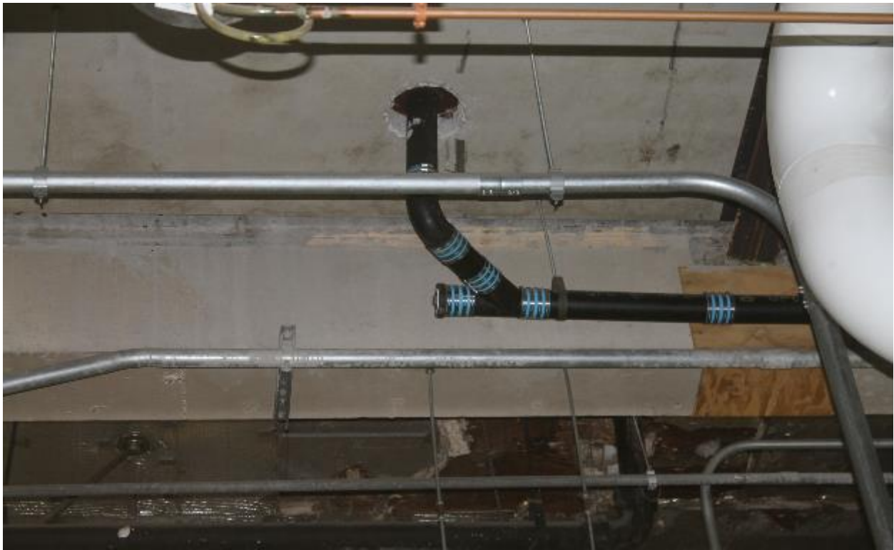
Photo 14: Boiler plant roof drain
