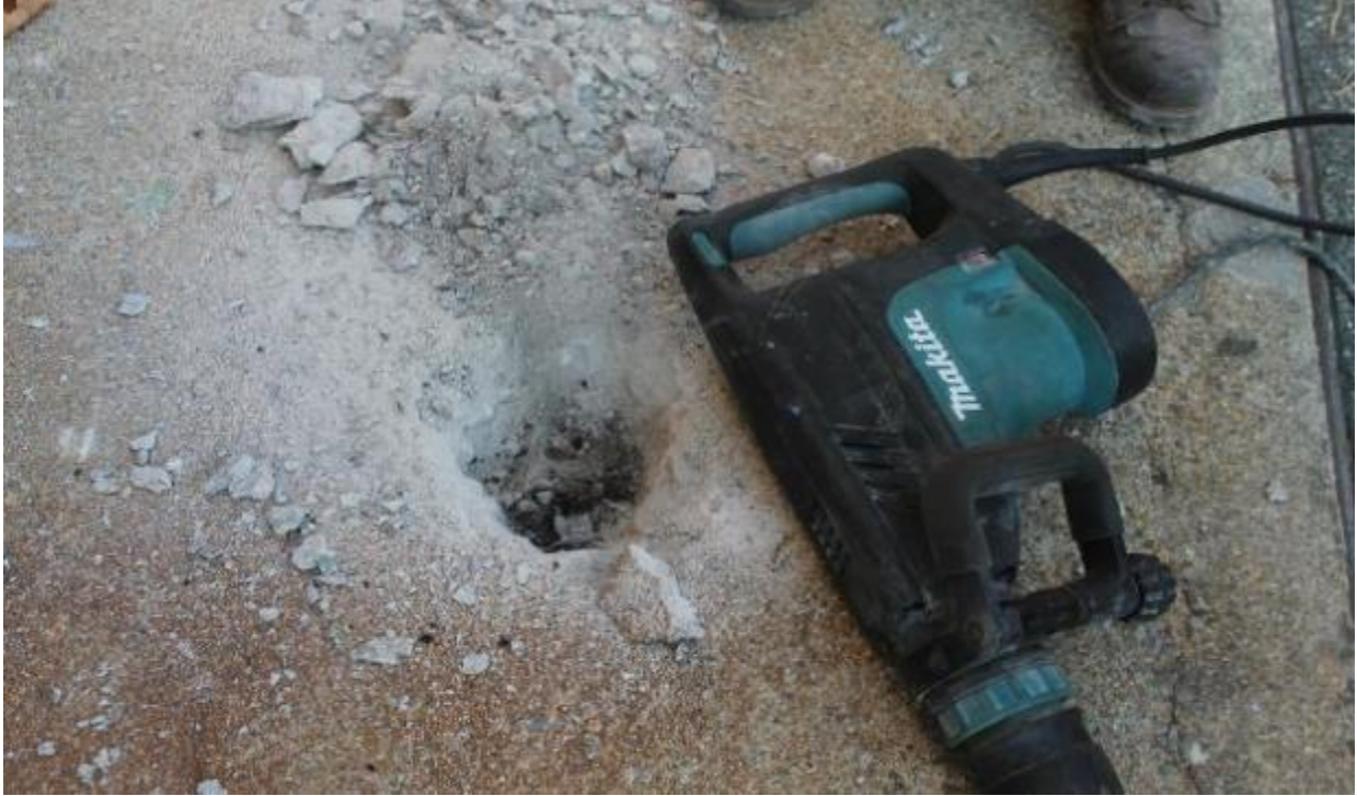
Photo 1: Black tar under sidewalk
