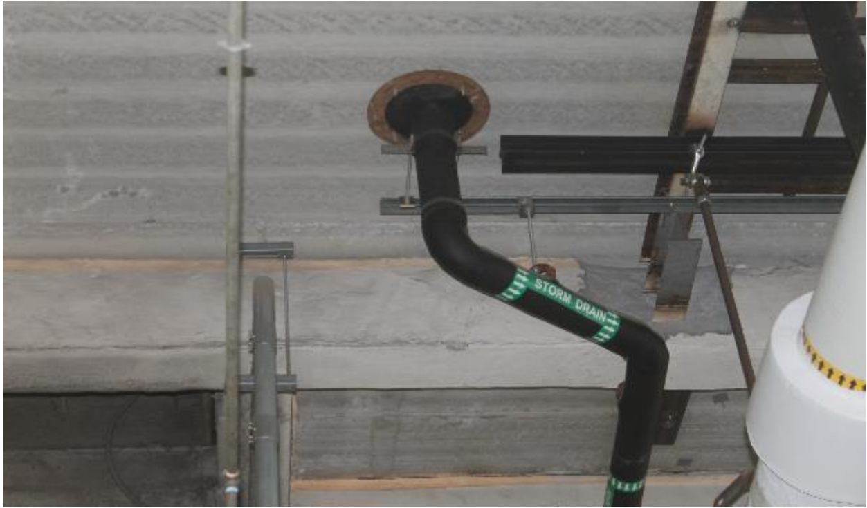
Photo 13: Boiler plant roof drain
