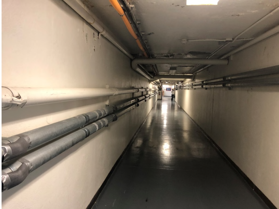
Main Corridor. Note skim on wall, grey epoxy wall/ceiling, and brown cove base/ adhesive
