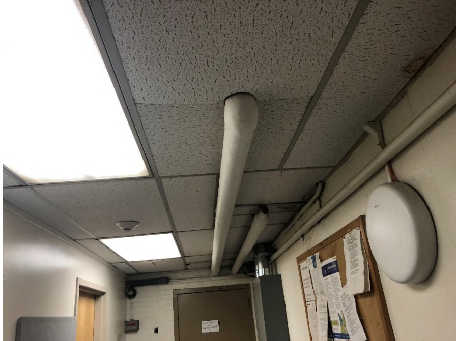
ACM pipe insulation in Adjoining Corridor
